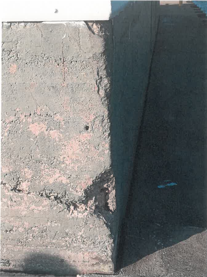
Northeast corner concrete foundation damage – full scale
