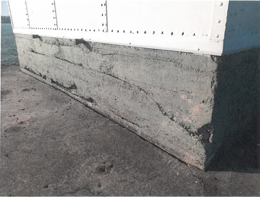
Eastern foundation face, from the northeast corner showing concrete damage
