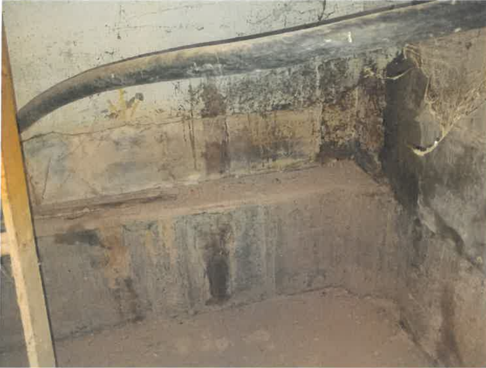
Interior view of SW basement, showing signs of long-term water intrusion – dried mud on floor
