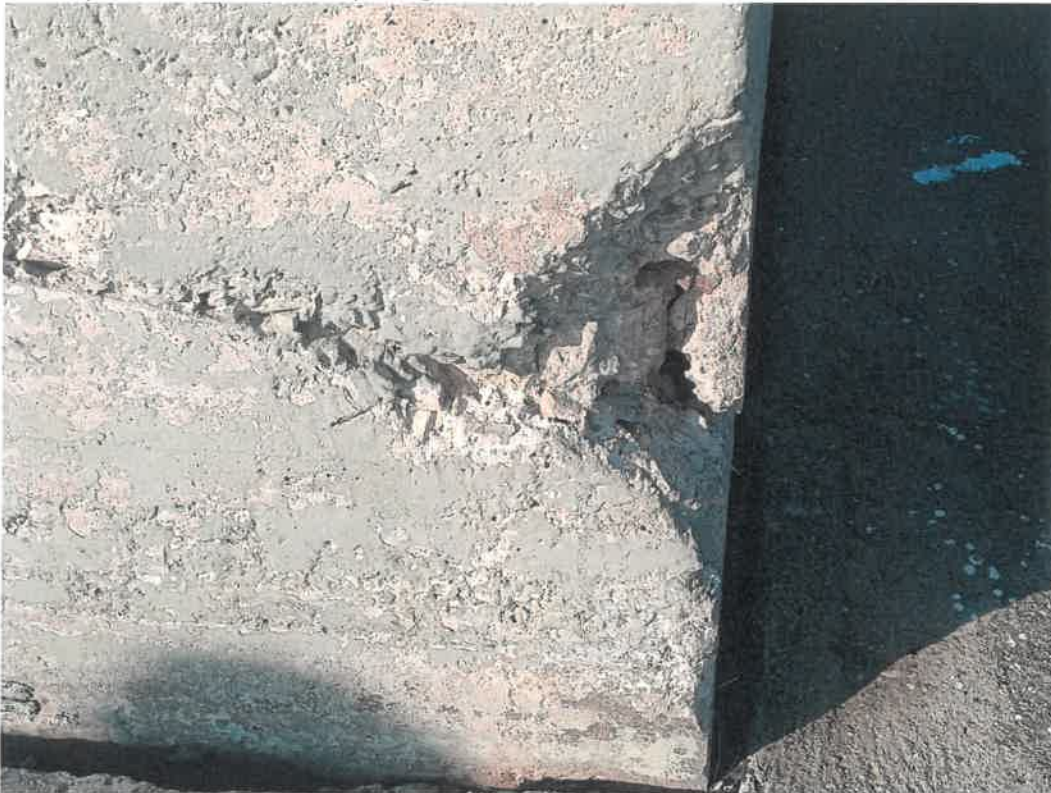
Northeast corner foundation damage
