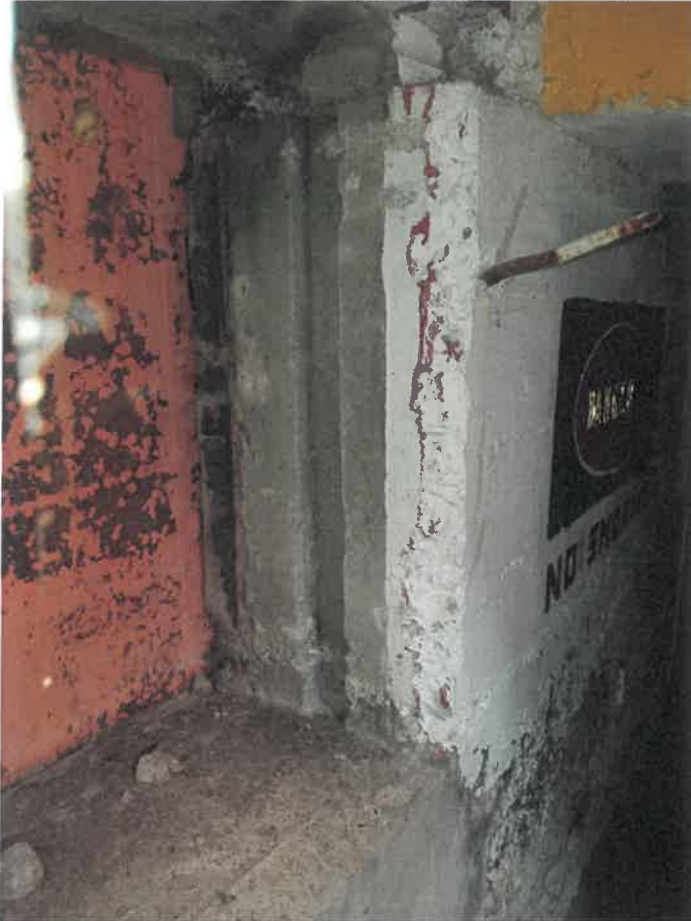
Interior west foundation wall, showing groove in concrete wall possibly from original mini door
