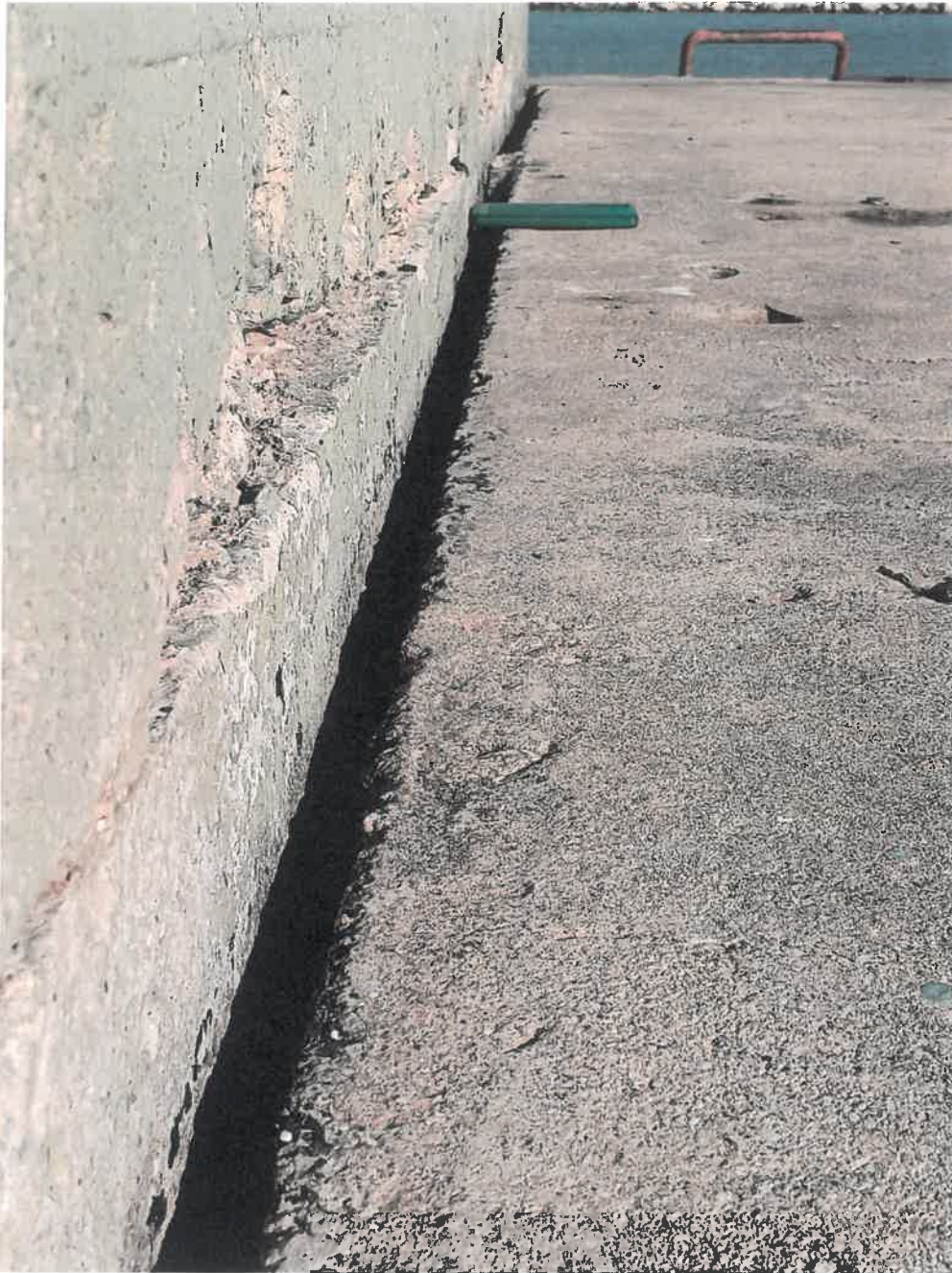
KLH east face – note missing mastic and concrete gap. Note smartphone shows gap width by comparison.
