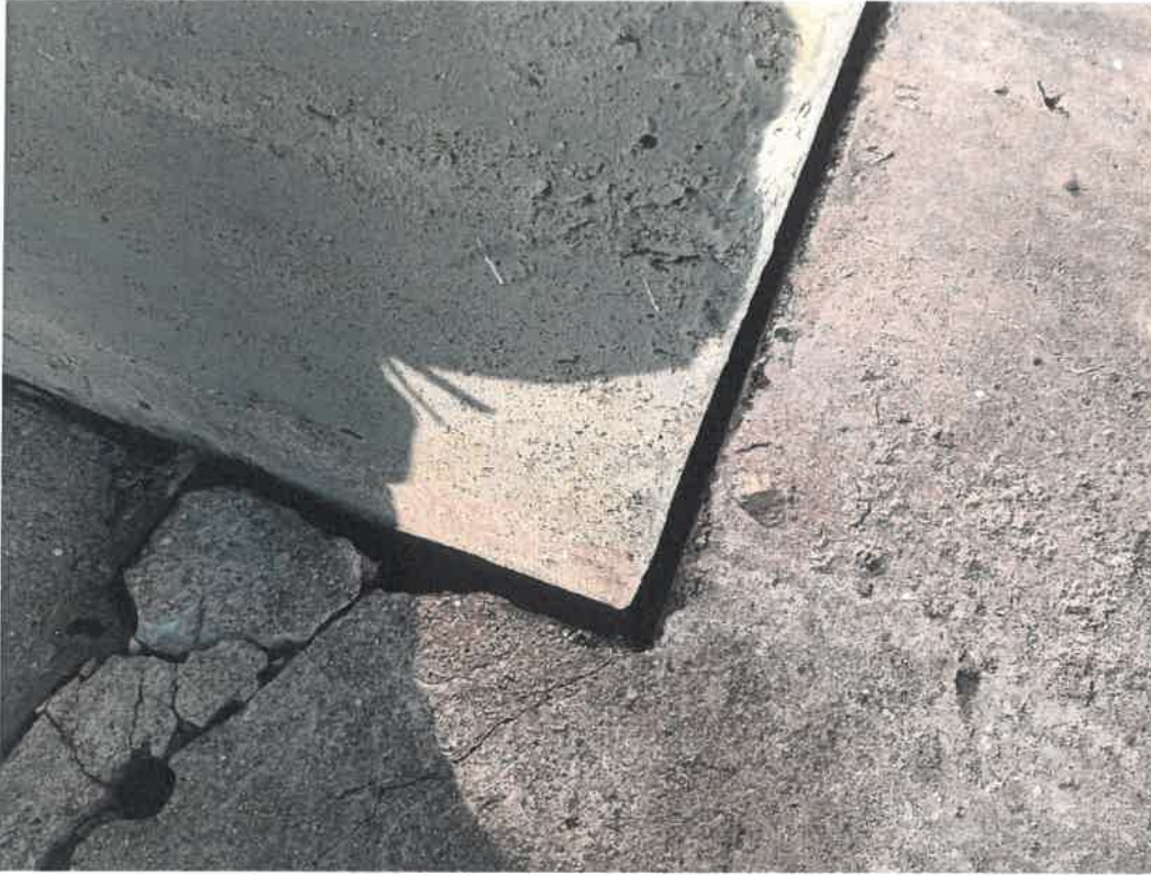
Northwest foundation corner, missing mastic
