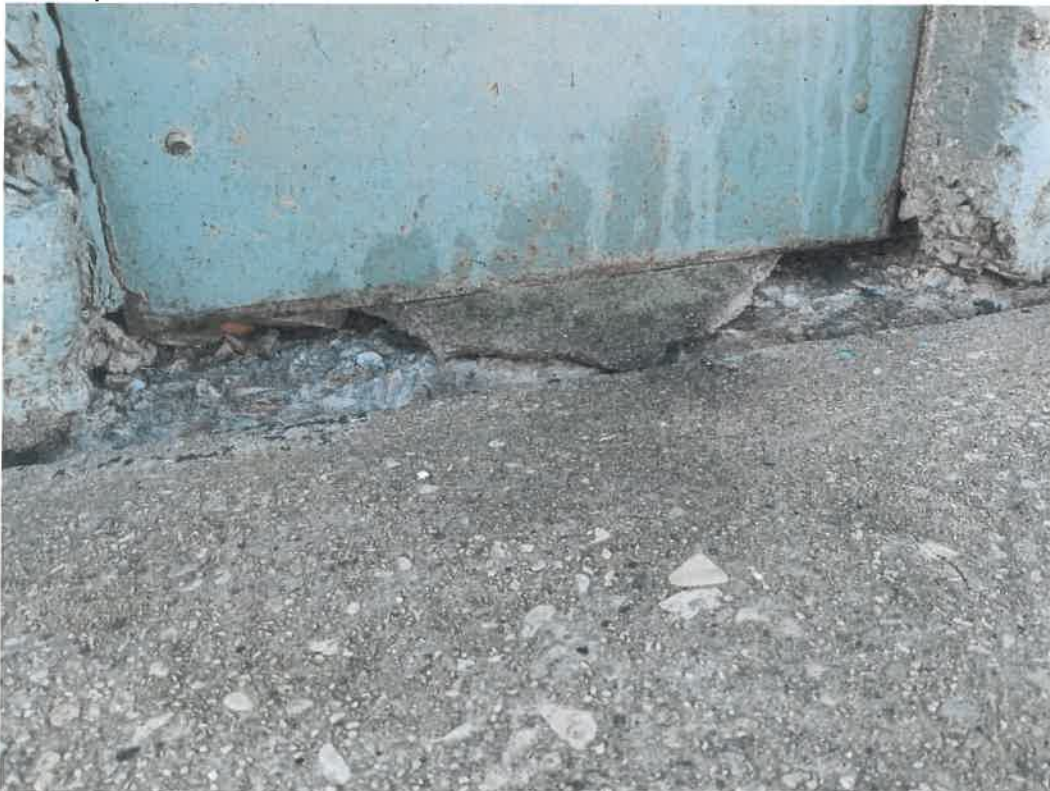
KLH damage concrete at exterior base exterior
