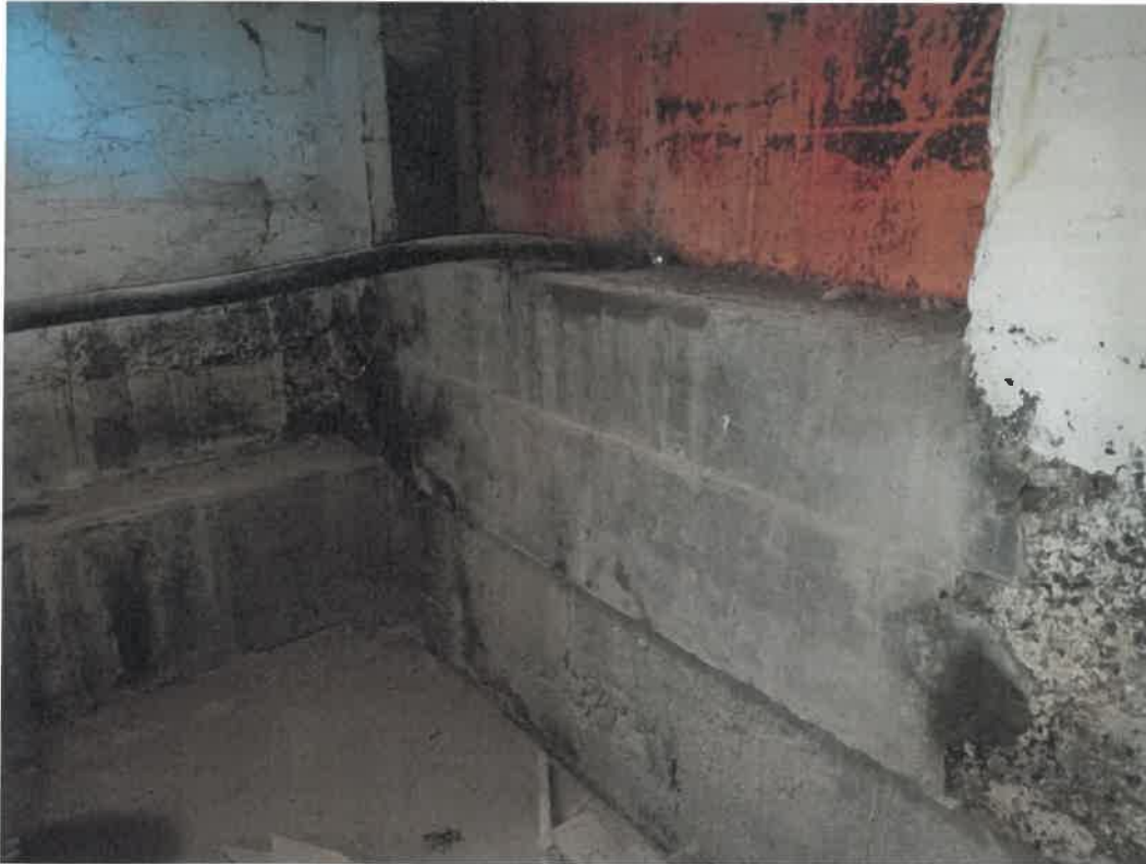
Wide view of SW foundation opening – see newer concrete under the metal plate. This is where the conduit entered the building when the lighthouse was automated.
